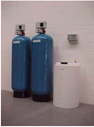
Softening and Filtration
